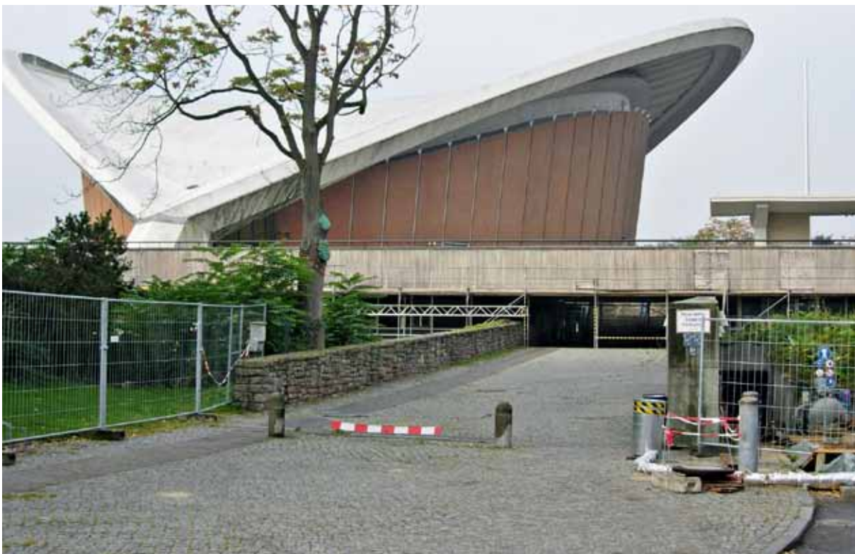
Carbon reinforcements were applied to structural components of the Haus der Kulturen der Welt und Kongresshalle (HKW) in Berlin
